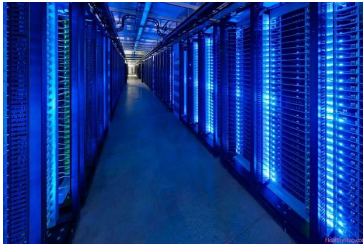
Figure 12. Data centers will become crucial to energy debate as “big data” increasingly drives business operations.
