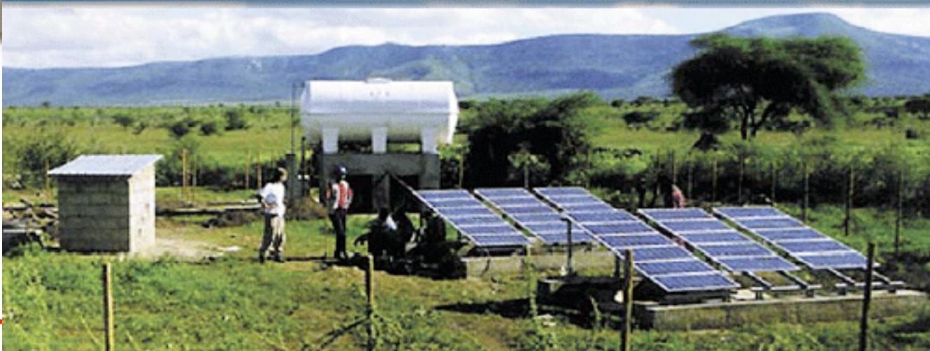
Photovoltaic Water Pumping System in Africa
