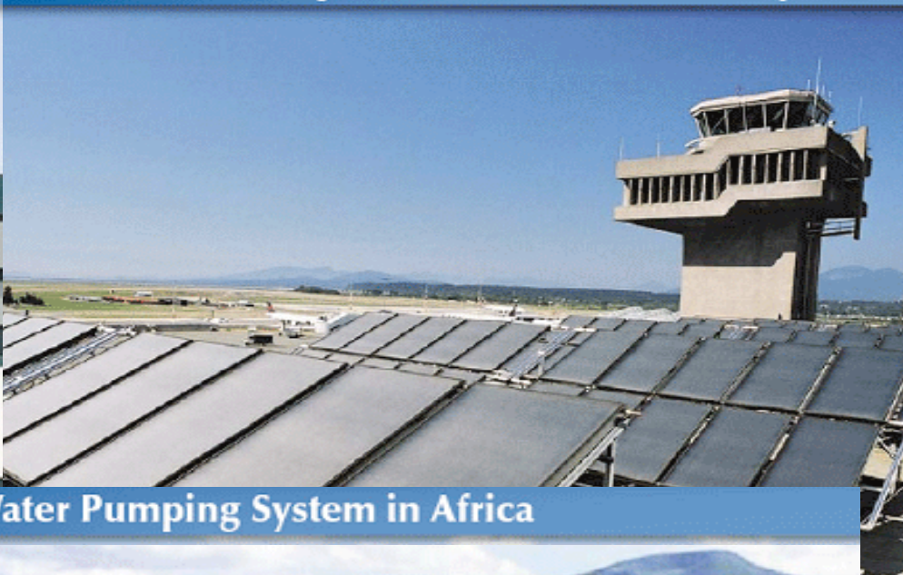
www.retscreen.net Solar Water Heating at Vancouver International Airport
