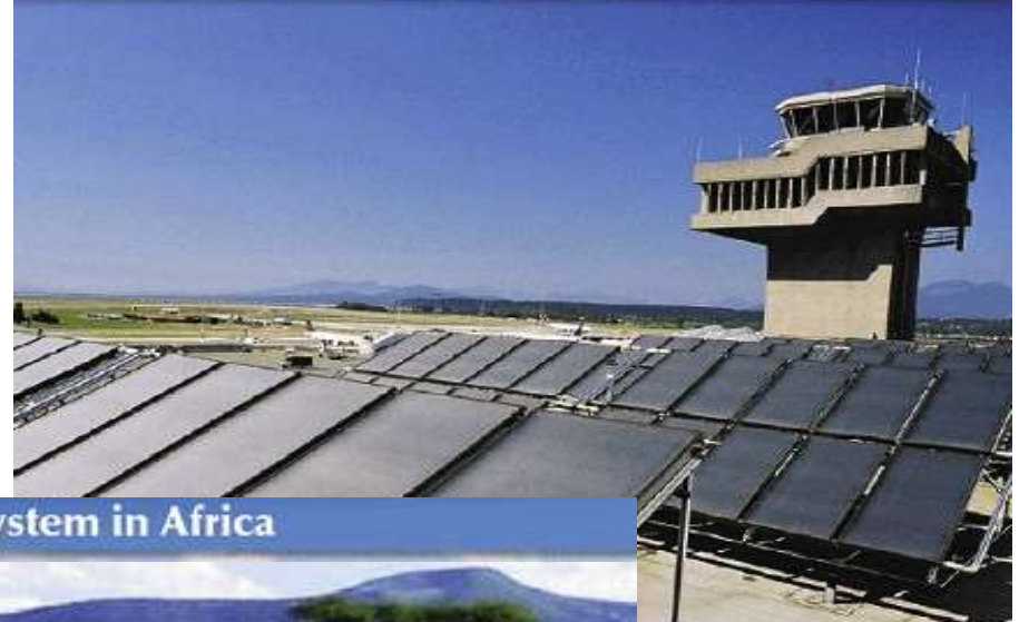
Solar Water Heating at Vancouver International Airport
